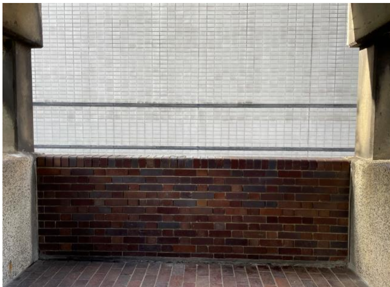
Mountjoy Close and incomplete Highwalk
